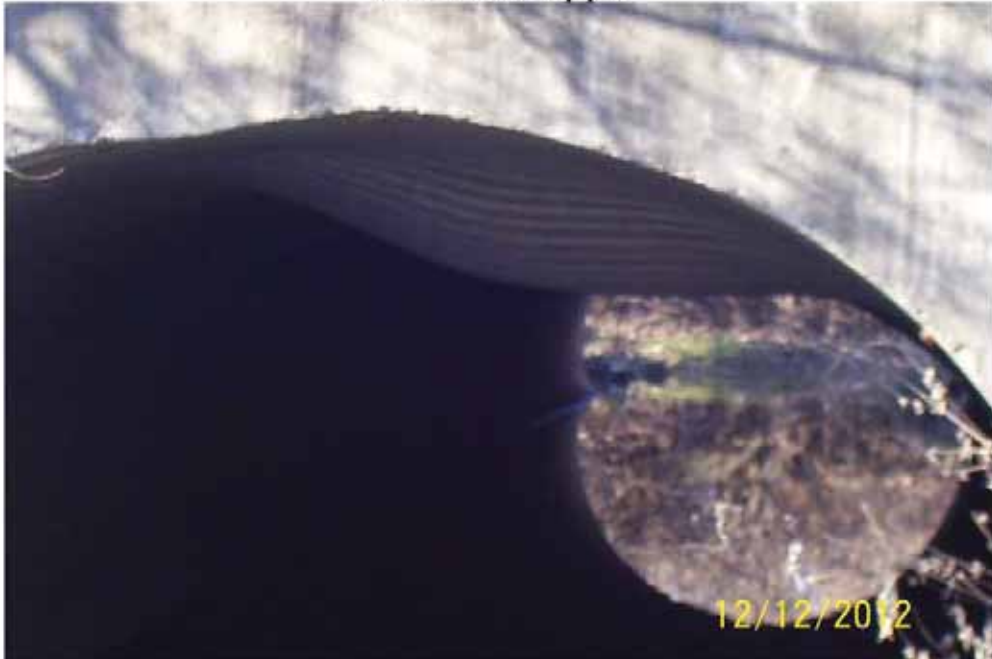
3607 Large deflection, East end of South pipe
